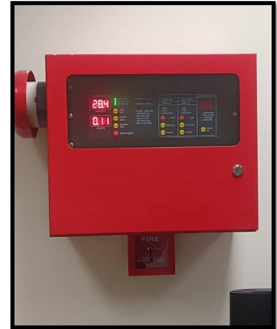
Fire Alarm Control Panel, FM 200 Bilik Server Aras 5 -PJH
