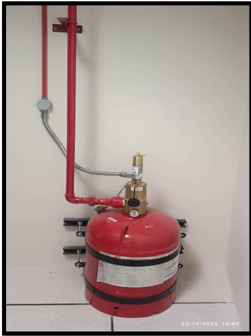
Fire Suppression System, FM 200 Bilik Server Aras 5 -PJH
